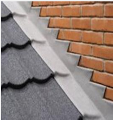
Cover lead in silver paint making it less attractive to thieves
