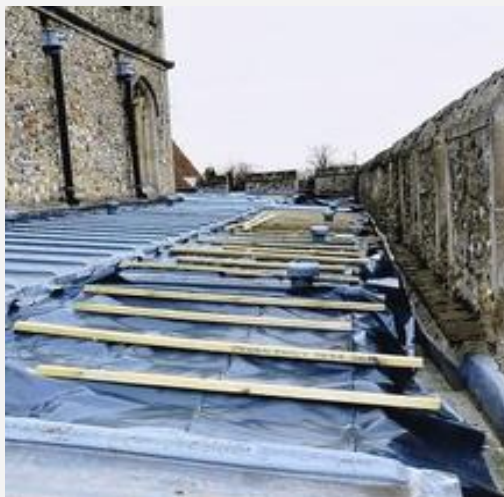
Check roofs so theft is discovered early before causing further damage
