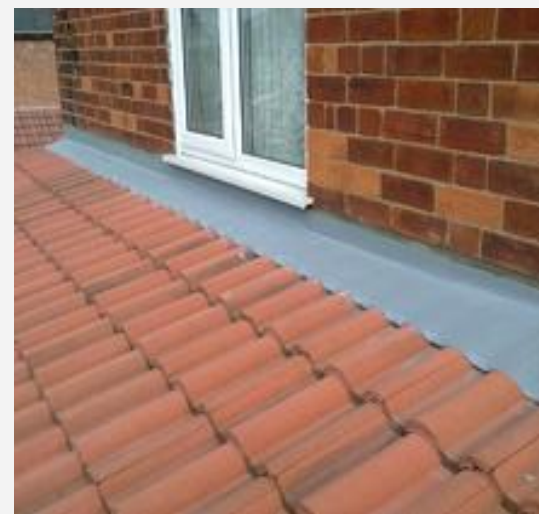
Replace lead with a substitute material when repairing damage
